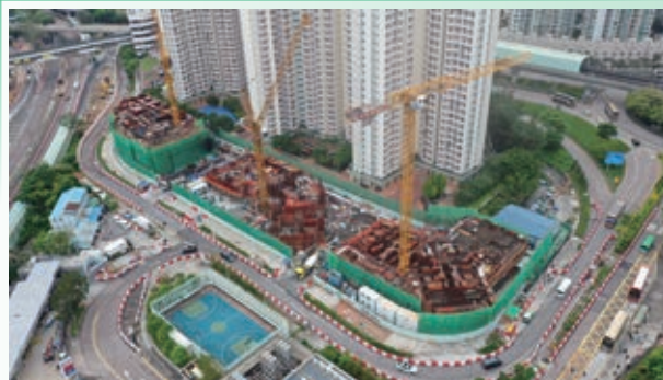
其中一个兴建中的绿置居2022项目—马鞍山锦柏苑 Kam Pak Court in Ma On Shan – one of the GSH 2022 developments under construction
