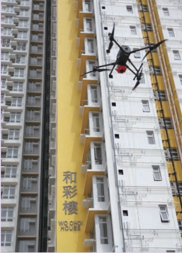
装上摄影机的无人机检查和田邨的外墙 A UAV with a mounted camera inspects external walls at Wo Tin Estate
