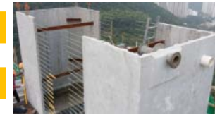
Precast Water Tank
