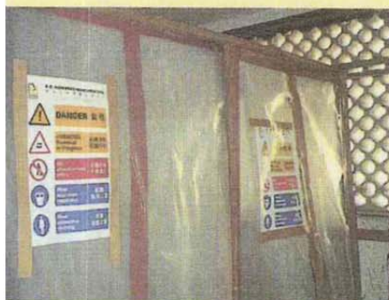
▲ Tarpaulin sheetings are in place to suppress dust releasing from the work site
