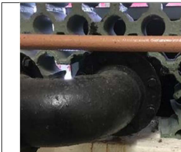
Disturbed grille panel
