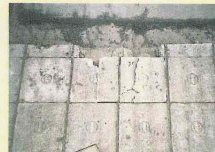
Roof tiles made of chrysotile (white asbestos) and cement
