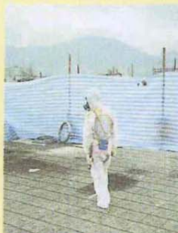
▲ A worker is taking air monitoring samples at the roof of a building from which roof tiles are being removed
