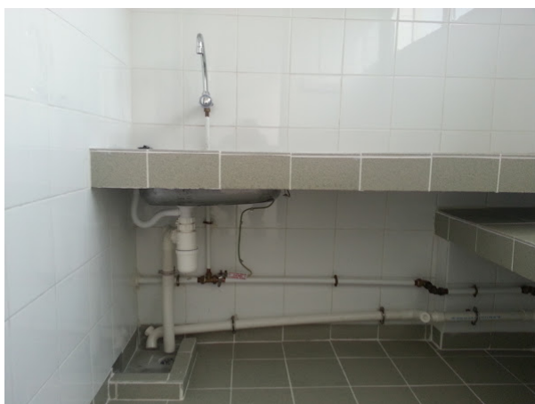
(b) Inside flat: copper pipes with compression joints
