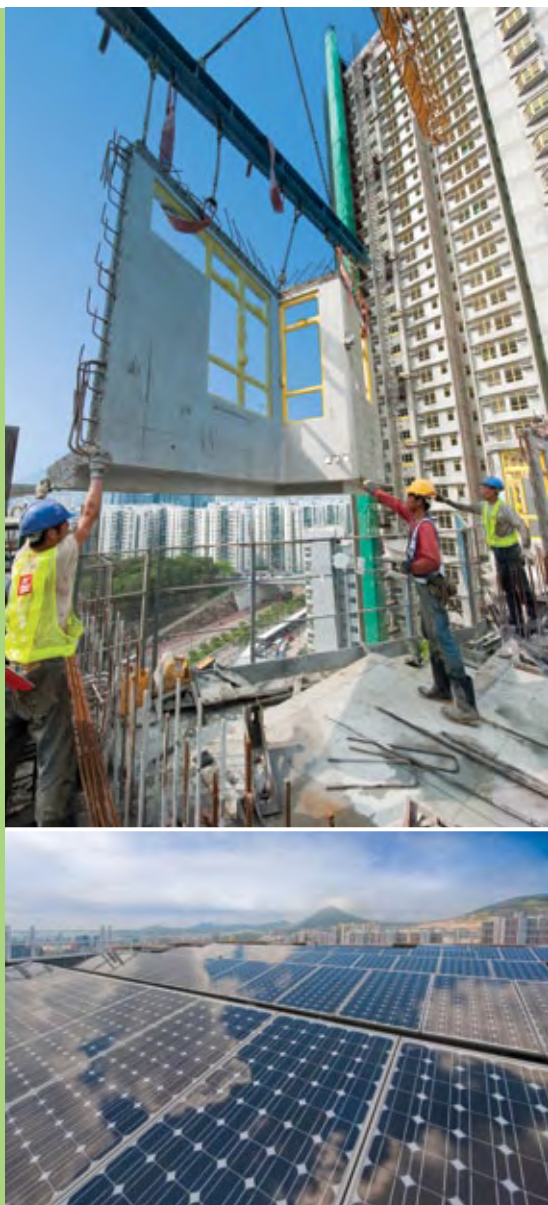
Top: One of our innovative green building techniques is the extensive use of pre-fabricated façades.
