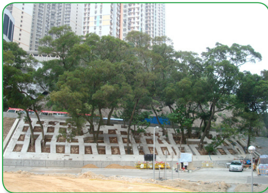
A slope at Sau Mau Ping is stabilised by soil nails and concrete grillages
