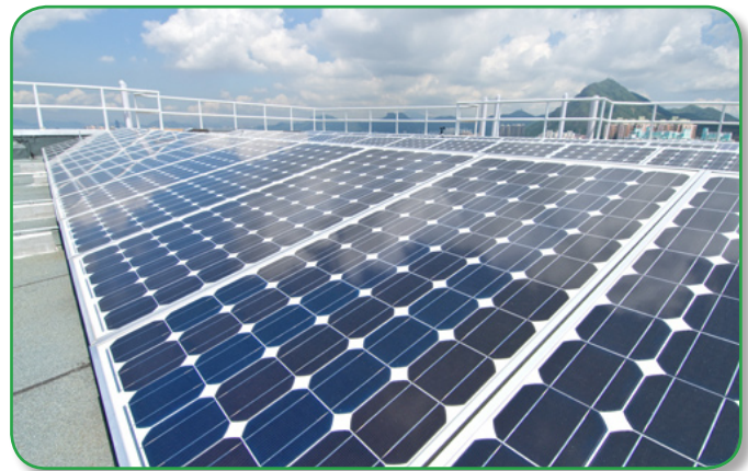
Solar panels of the PV system installed on roofs
