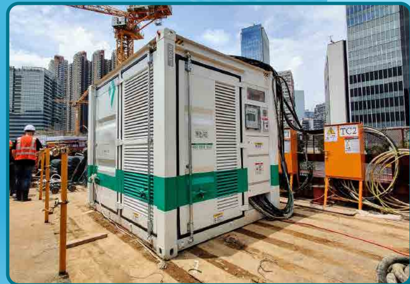
Battery Energy Storage System
