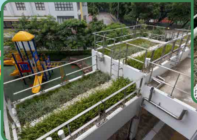
Green roof at Wui Chi House of Tung Wui Estate with ZIS application
