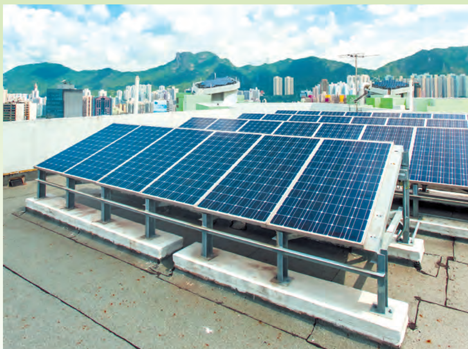
■ A grid-connected PV system.
