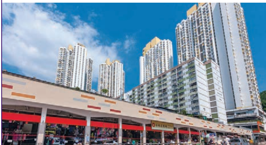
石硤尾街市的外牆改善工程前(上圖)後 Refurbishment of external façade of Shek Kip Mei Market – before (top photo) and after
