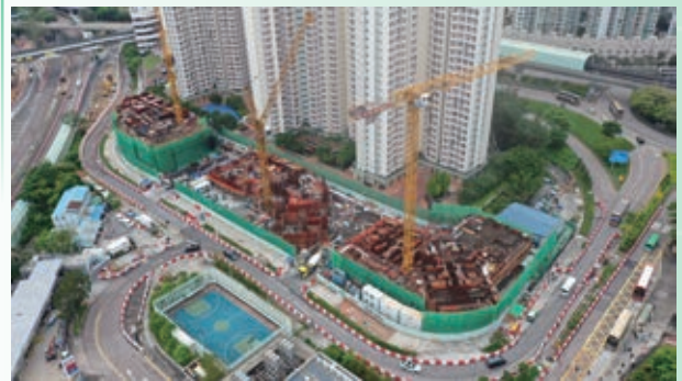
其中一個興建中的綠置居2022項目—馬鞍山錦栢苑 Kam Pak Court in Ma On Shan – one of the GSH 2022 developments under construction
