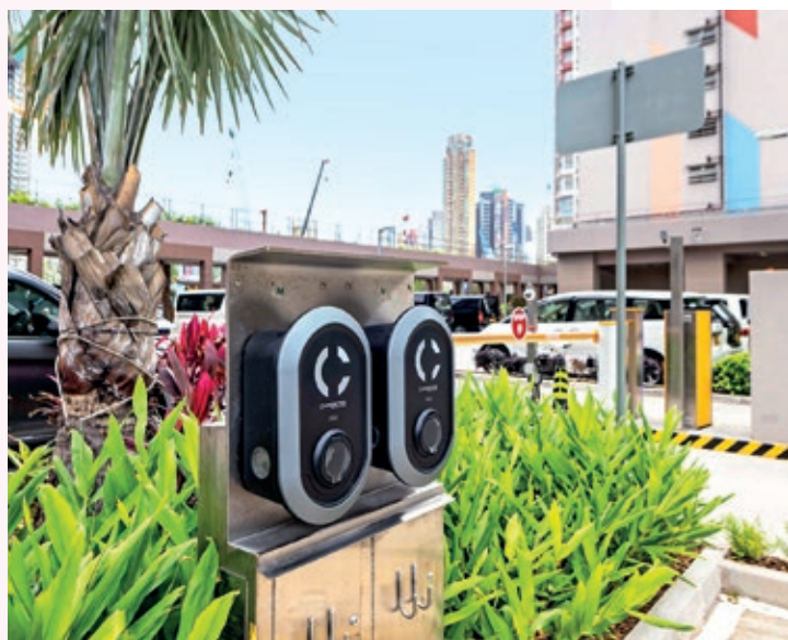
启德启欣苑的电动车中速充电器 Medium chargers for EVs at Kai Yan Court in Kai Tak
