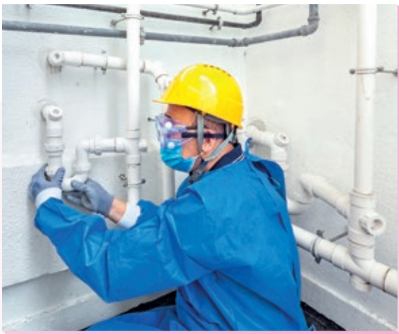
排水管改善计划为居民检查和改善排水系统 The DEP includes inspection and improvement works in estate drainage systems
