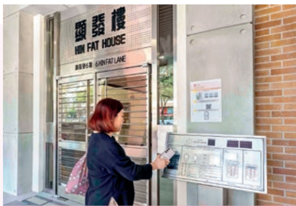
智能卡门禁系统令居民出入更安全快捷 The Access Control System offers safe and convenient access for residents
