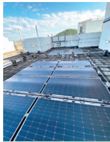
东区小西湾邨的柔性太阳能光伏发电系统 A flexible PV system at Siu Sai Wan Estate in Eastern District
