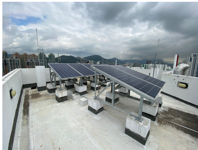
PV Panels at Hoi Ying Estate
