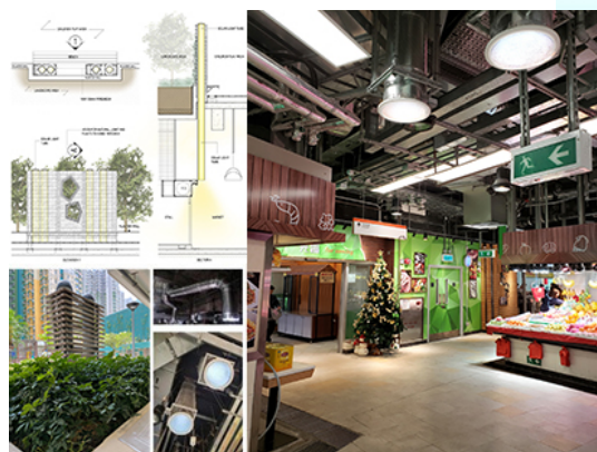
To better utilise natural light to reduce energy use, a total 30 solar light tubes are installed at On Tai Estate for lighting up wet market and car park.
