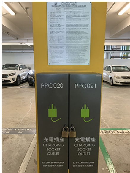
EV charging facilities at Choi Hing Court, Kwun Tong
