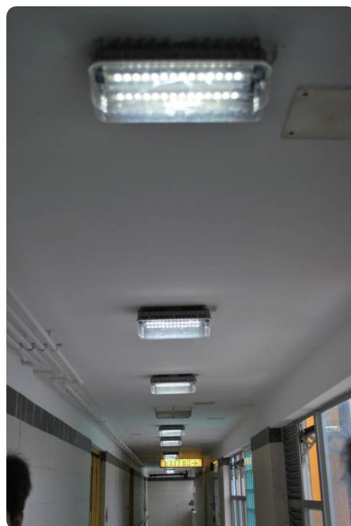
Corridor Using LED Bulkheads
