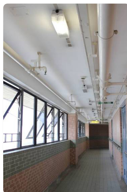
Modified Lighting Circuits in Corridor Allow Switching off Lights Selectively in Daytime in Ho Man Tin Estate
