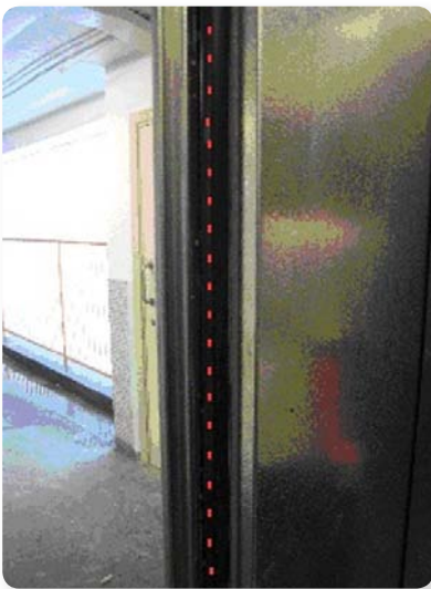
Infra Red Detection Beams at Lift Car Door
