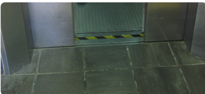
Black and Yellow Warning Strips on the Apron Sheets of Lift Car
