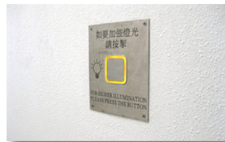
Manual push button of two-level lighting control system
