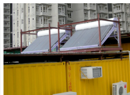
Provision of solar hot water heaters in workers' shower area
