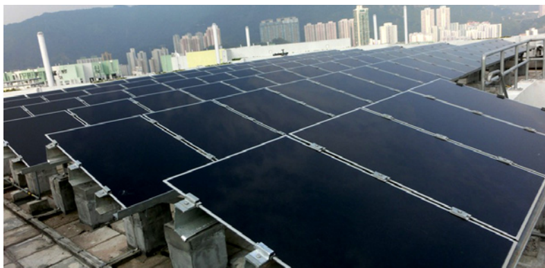
Solar panels at Kai Tak Site 1B
