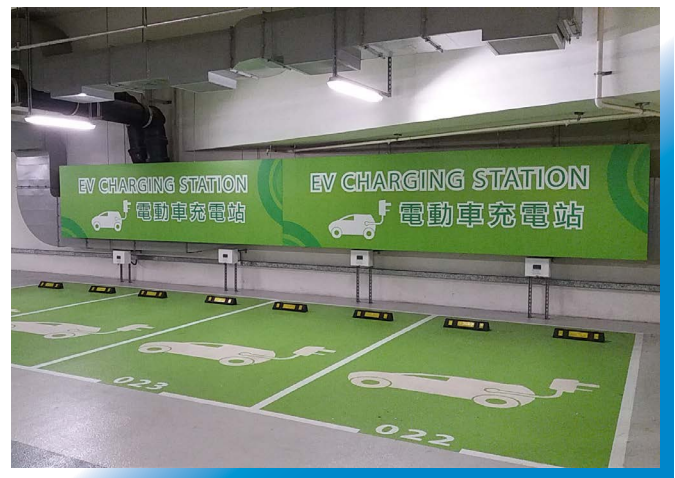
▲ EV Charging Station
