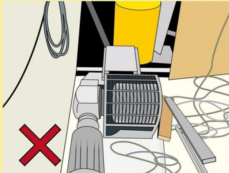
Improper Guarding on Electrical Winch 電器絞盤保護不當
