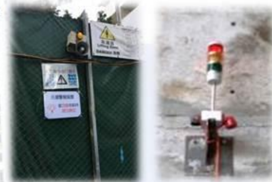
Audio Visual Lifting Alarm System & Automatic Safe Load Indicator
