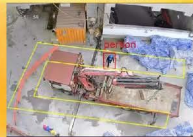
Danger Zone Alert
