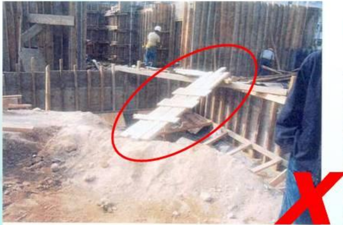
Unsafe access to formwork area
