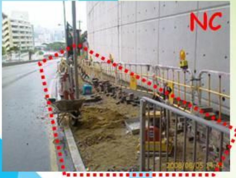
No continuous pedestrian barriers
