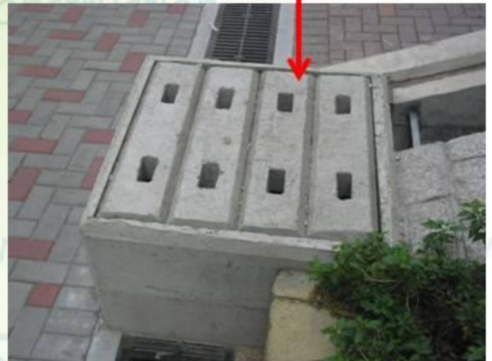
Catchpit covered up with concrete strips
