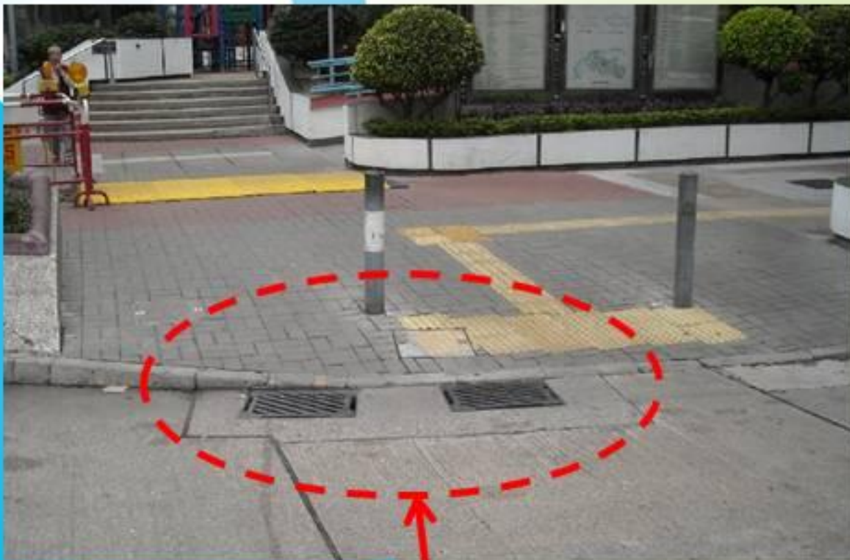
Gullies in front of crossing
