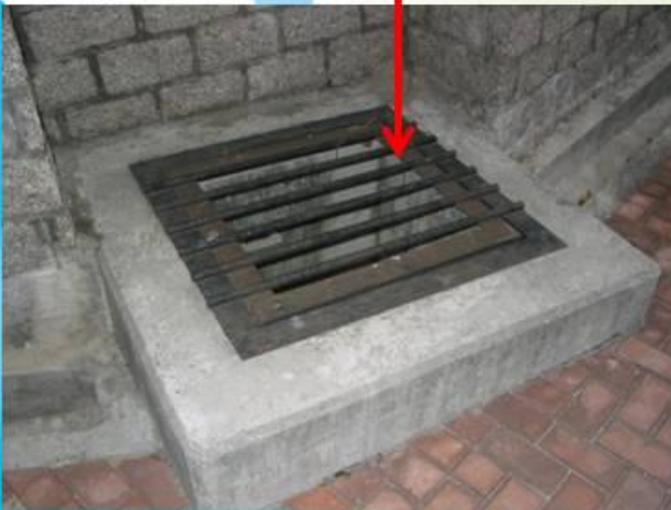
Catchpit with gratings
