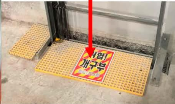
Fibre Board at Floor Opening
