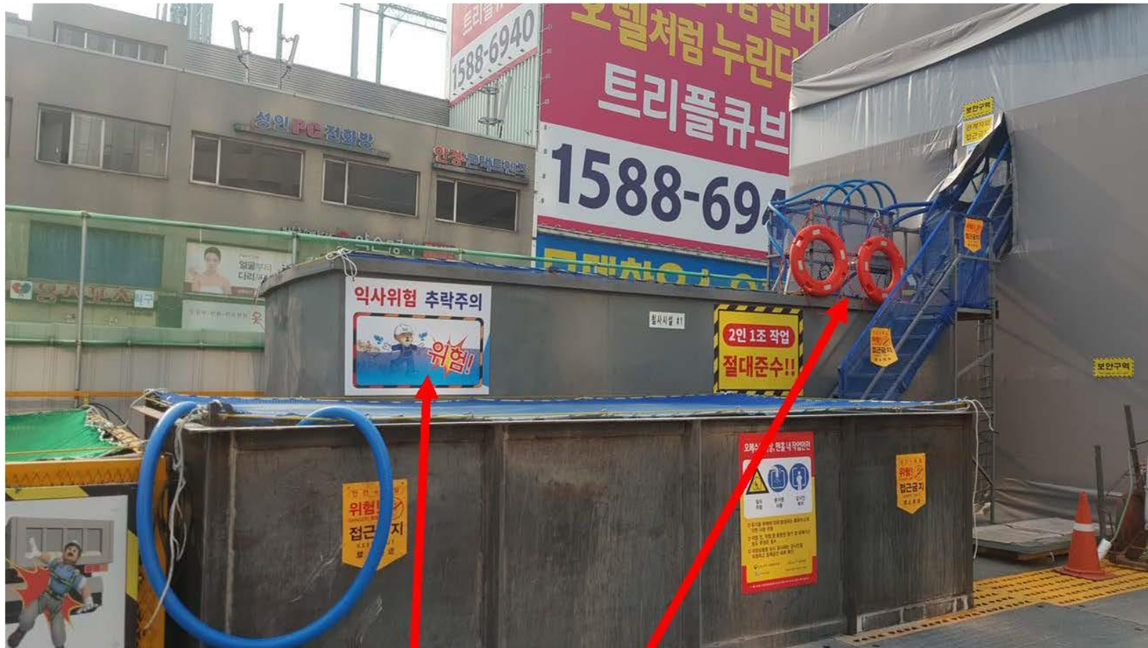
Safety Notice & Measures next to Water Tank
