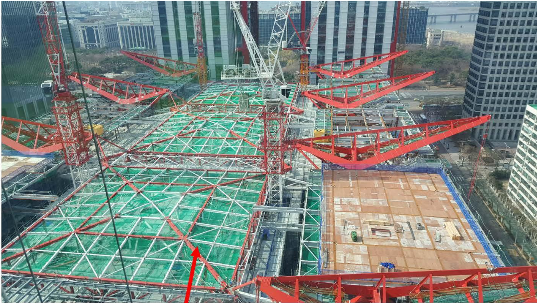
Fall-arrest System at Steel Roof
